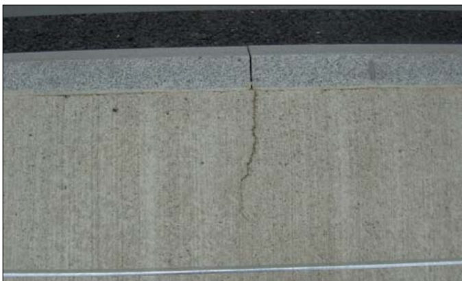
FIGURE 5 & 6 Cracks on the drainage areas
