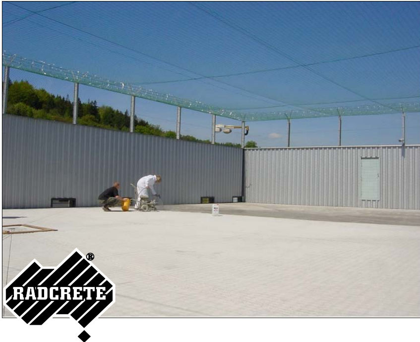
FIGURE 1 Radcon Formula #7 application onto a rooftop area of the State Prison in Czech Republic.
