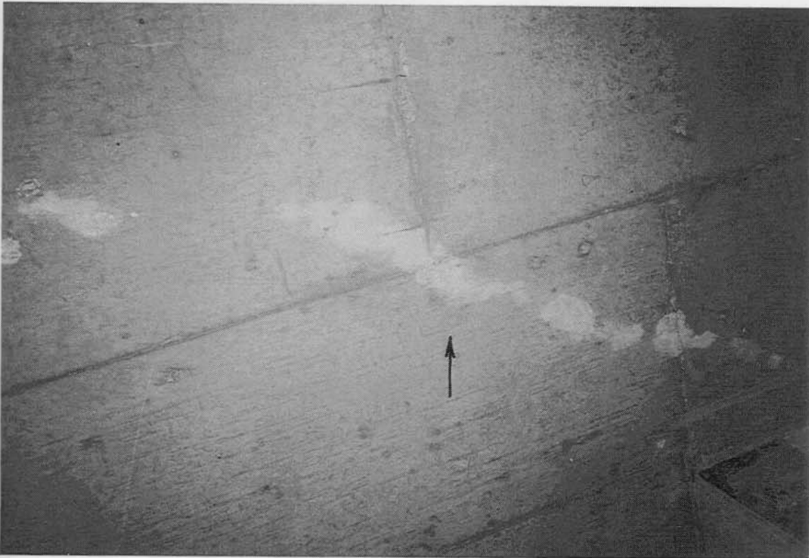
Photograph 21: View of soffit after test, (30 minutes). Note no evidence of water penetration.
