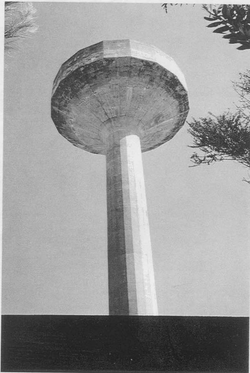
Photograph 13: View of tank showing cold joints
