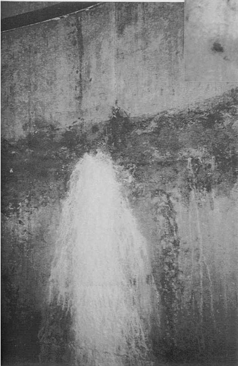
Photograph 15: View of weeping construction joint from inside tower. Note large build up of Calcium deposits.
