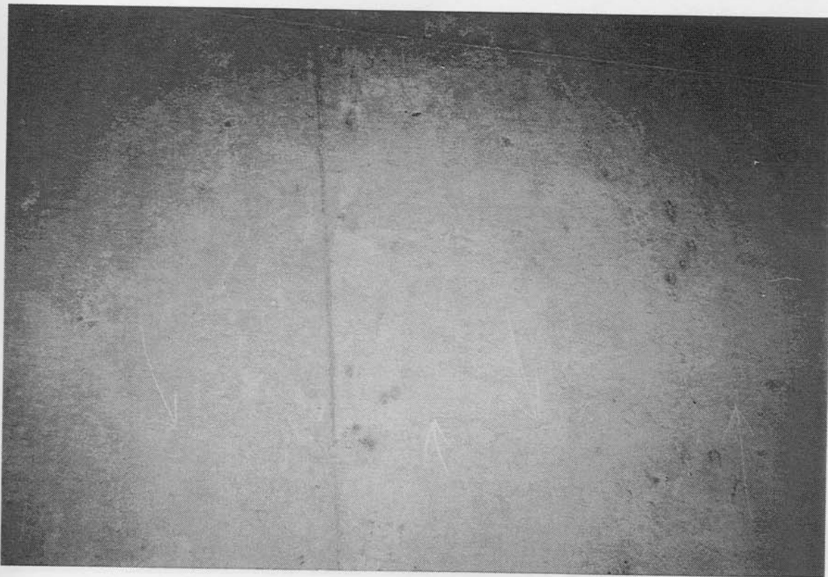
Photograph 6: View of soffit showing mid span crack, Note no water marks.
