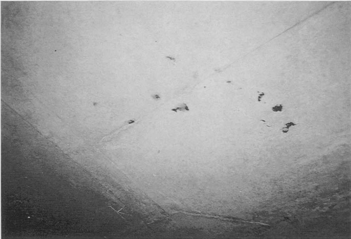
Photograph 12: View of soffit showing dampness in poorly compacted area.
