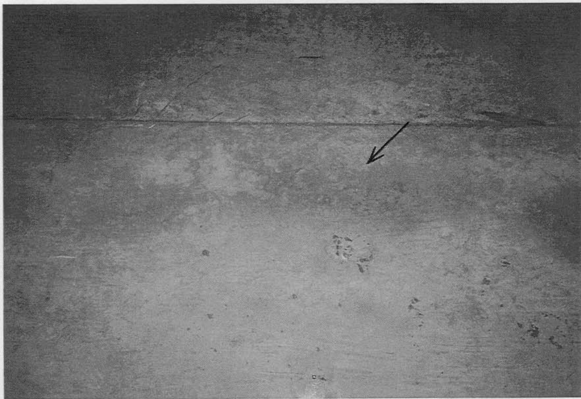
Photograph 18: View of soffit after test, (30 minutes). Note no evidence of water penetration.
