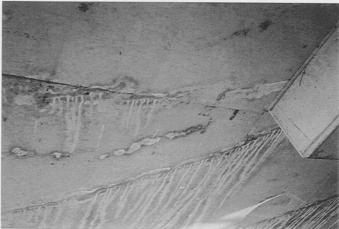
Photograph 6: View of soffit showing mid span crack. Photograph 3: View of soffit after ponding test, (30 mins)
