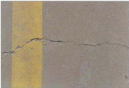
FIGURE 30 - ONE OF MANY CRACKS IN THE DECK
